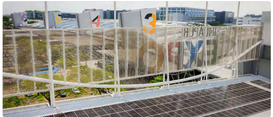
Over 17,000 photovoltaic panels installed on the rooftops of 10 exhibition halls and convention wing at Singapore EXPO, Singapore's largest purpose-built MICE facility.
